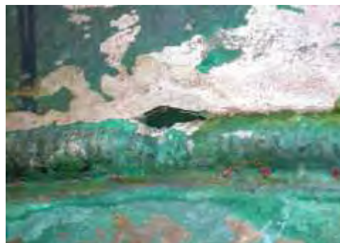
Figure 1: Example of galvanic corrosion (in this case dissimilar weld corrosion in heat affected zone)
